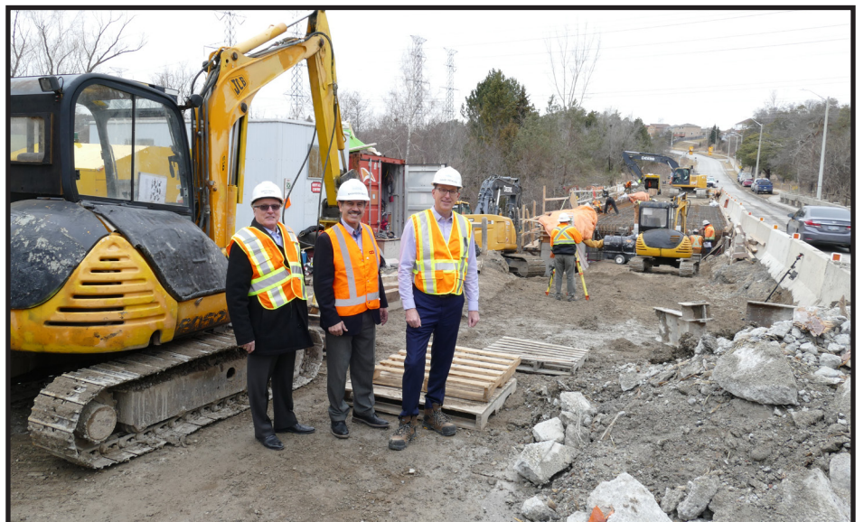
Mayor Ryan and Councillors Pickles and Butt check in on the progress of the reconstruction of Palmer Bridge on Valley Farm Road.
